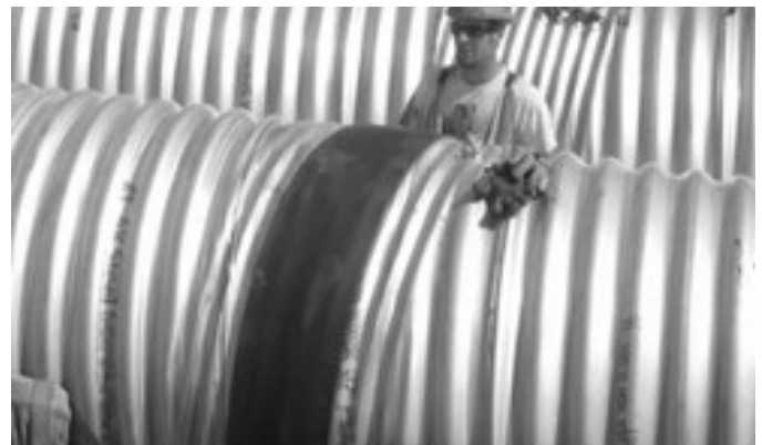
After the second pipe is placed, the half of the rolled gasket is placed over the second pipe.
