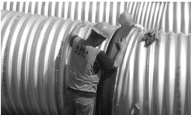
Sleeve gaskets are installed by putting one half of the gasket on the first pipe in the trench, then rolling the other half gasket over.
