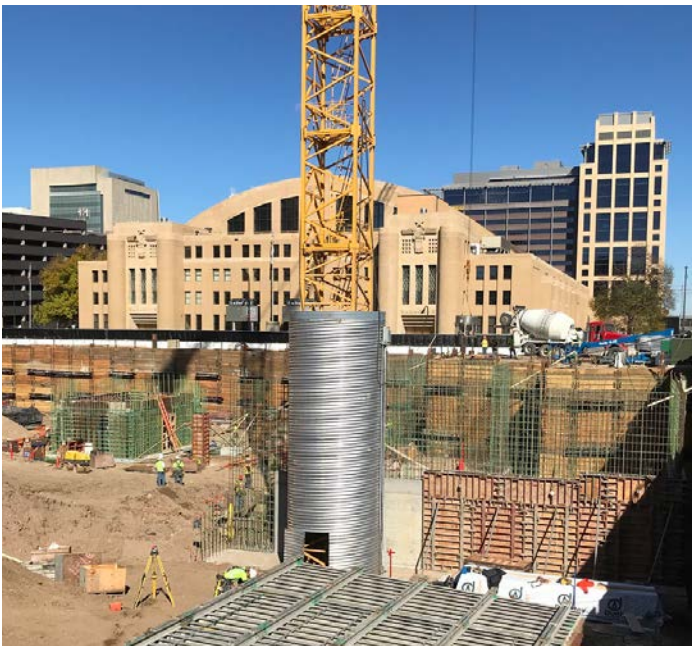
144" diameter HEL-COR® 5 x 1 Corrugated Steel Pipe used as a crane tower enclosure during the construction of a parking garage in an urban area.
