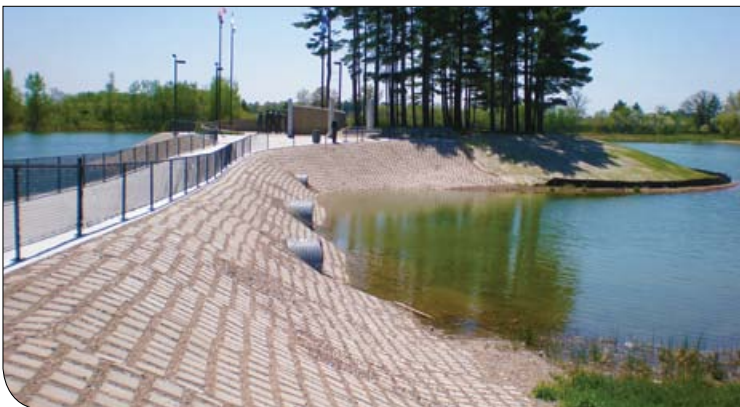
Korean War Veterans Memorial (WI) – replacement of cast-in-place concrete on Memorial causeway and reinforcement of the shoreline (ArmorTec)
