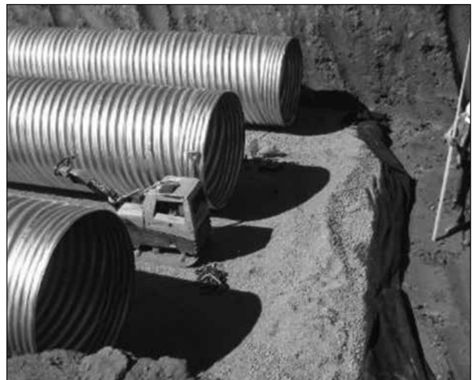
Culvert foundation required undercutting and importing 18" of granular fill for pipe bedding.
