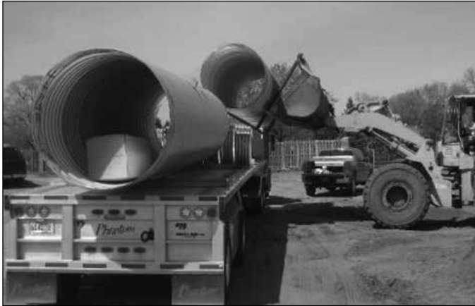
Lifting CMP off the flatbed with a front end loader and forks
