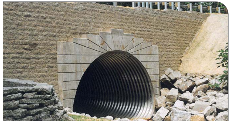
Bath Township (OH) – emergency replacement when flooding washed out a 100-year-old stone arch (ALSP)
