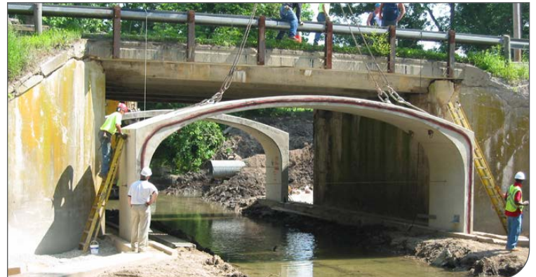
Dayton-Springfield Road (OH) – precast system installed under existing beam bridge to reduce road closure (CON/SPAN)
