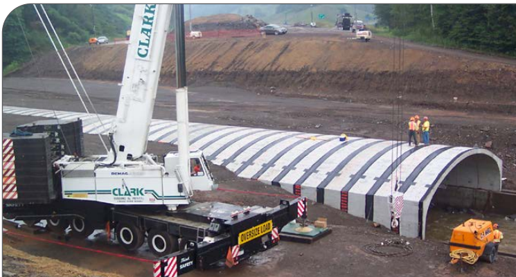
Interstate 88 (NY) – emergency replacement for DOT when storms washed out highway (CON/SPAN)
