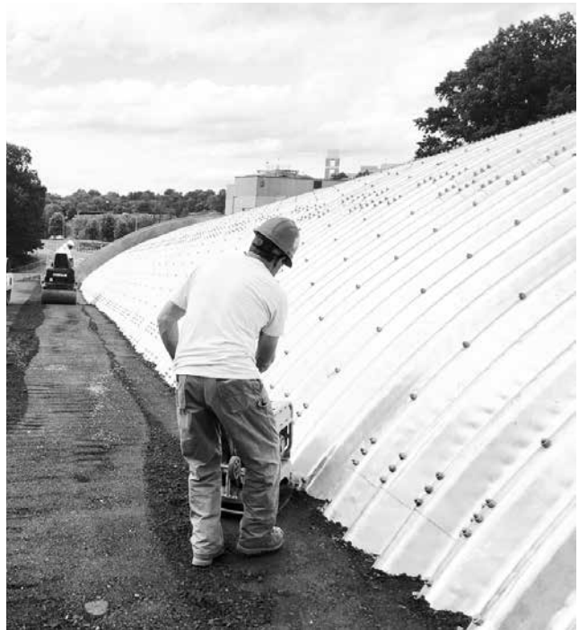
Each lift shall be compacted to a minimum 90% density per AASHTO T-180.
