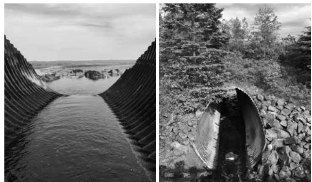
Bay of Fundy | Robinston, ME 52-Year-Old Aluminum Structural Plate Installed in 1966 | Inspected in 2018
