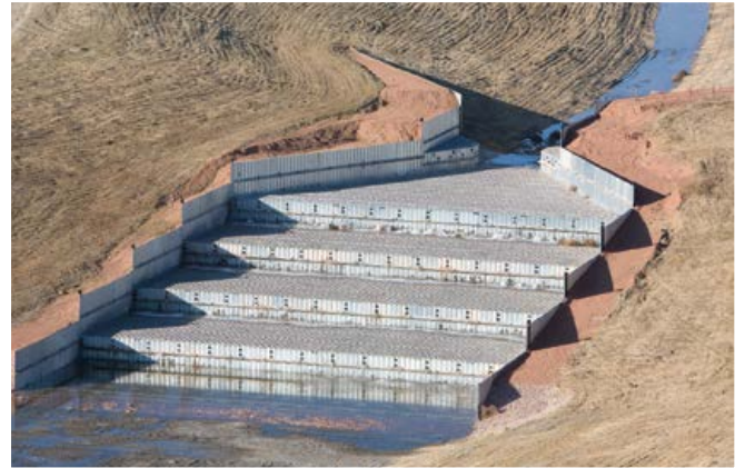
Combination solutions including metric sheeting and A-Jacks or ArmorFlex create efficient grade change structures for water conveyance.
